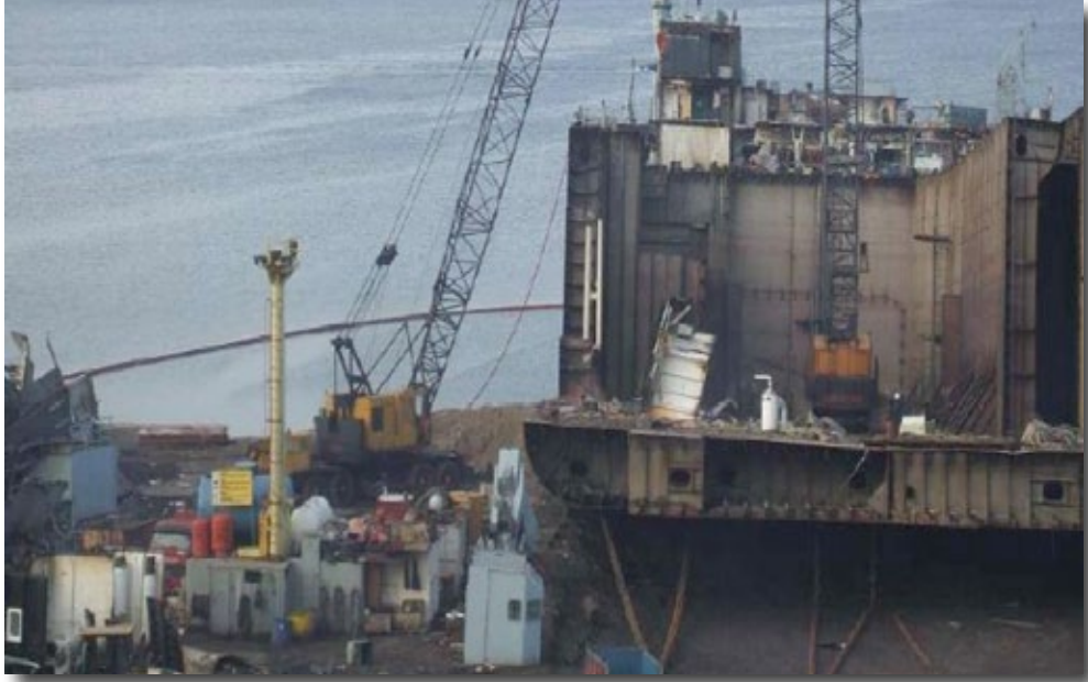
Deck 3 prior to being cut & removed Heavy Machinery is used to remove large pieces of the vessel for processing
