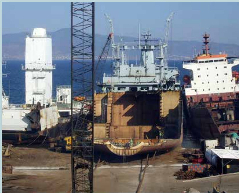
Progress of dismantling of works at the (Beg Oct) To the left of Ex-RFA Bayleaf is Ex-HMSTrials Barge Longbow which was also sold to LEYAL in Aug 2012
